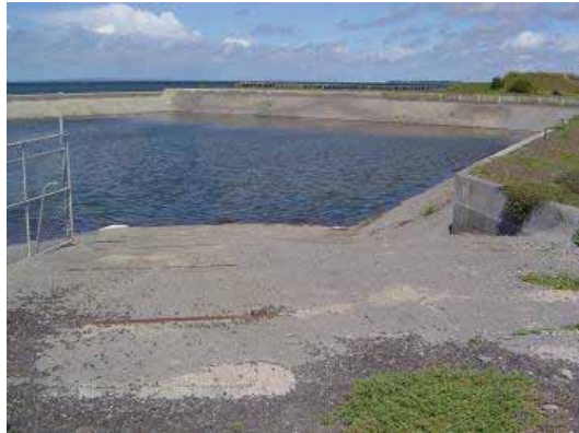
Photograph E.0.14 Horizon Tank (Woodhead International, 2004)
