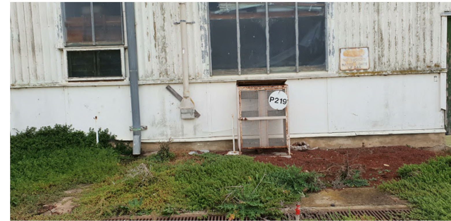
TYPICAL DETERIORATION OF EXTERNAL CLADDING
