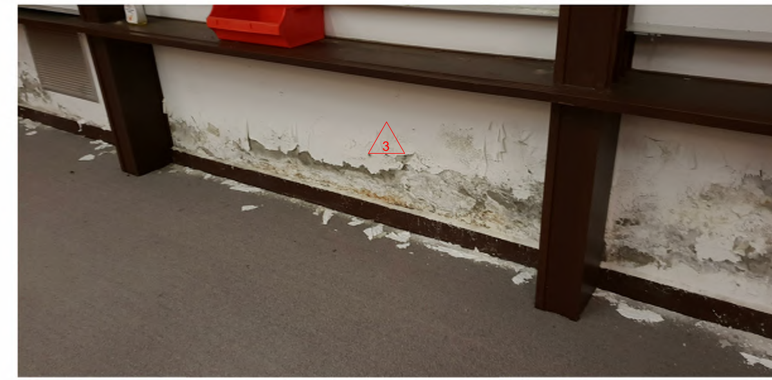
SCOPE 3 - IMAGE OF DAMAGED INTERNAL WALL TO THEATRE
