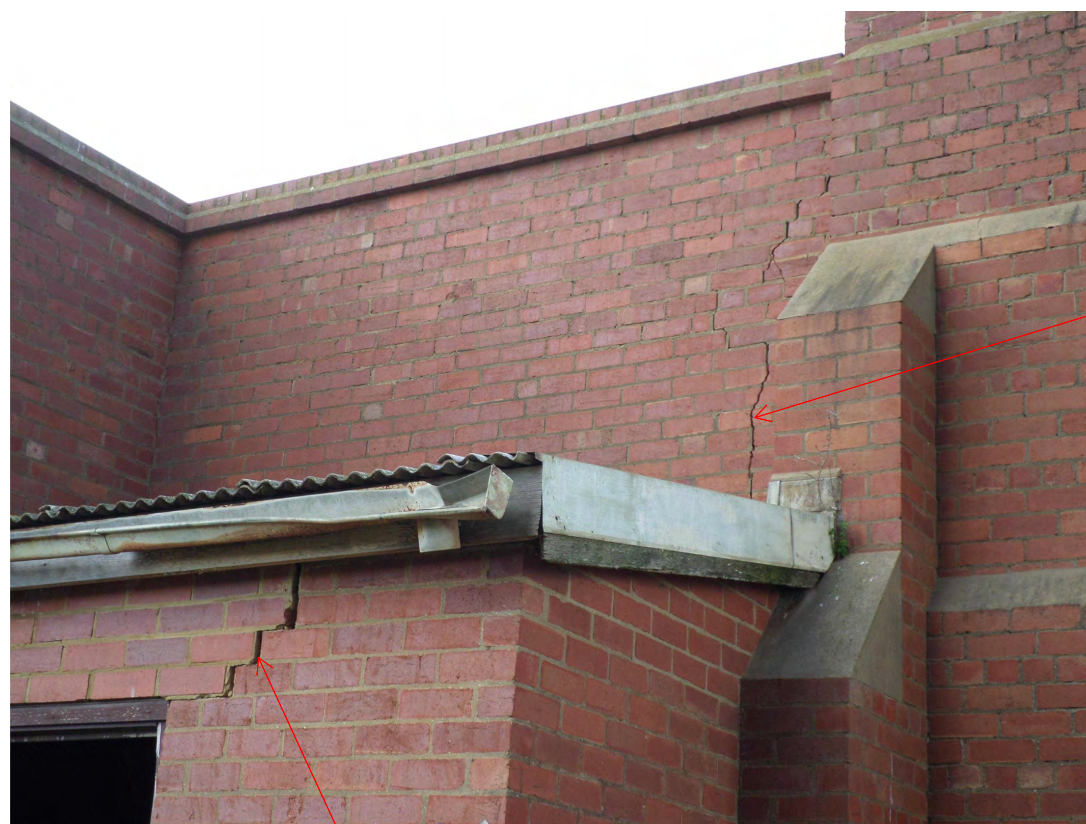
Exposed brickwork cracks
