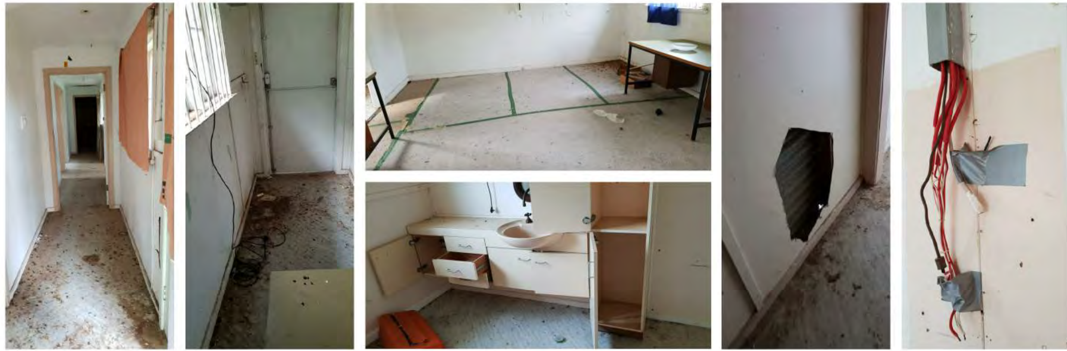
IMAGES OF TYPICAL DETERIORATION
