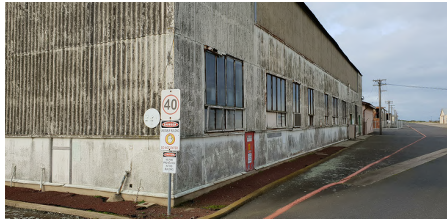
DETERIORATION OF EXTERNAL CLADDING - TYPICAL
