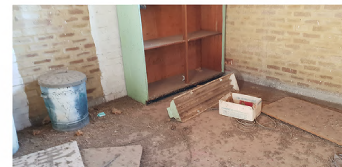
IMAGES OF TYPICAL DETERIORATION
