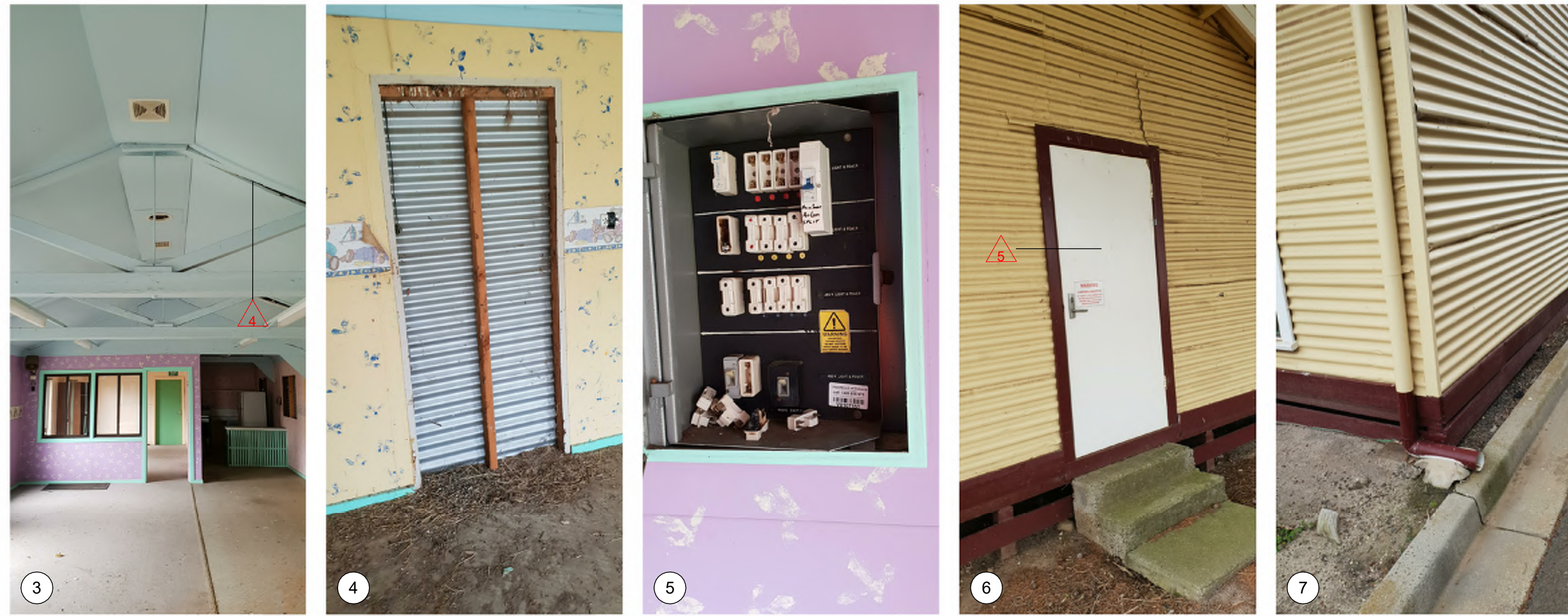
IMAGES OF TYPICAL DETERIORATION
