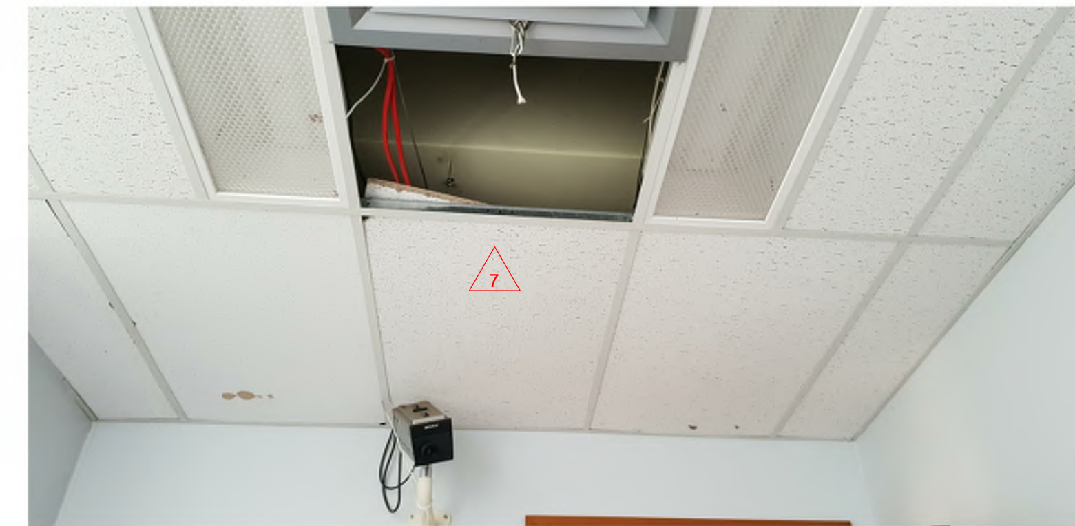
MISSING AND DAMAGED CEILING TILES
