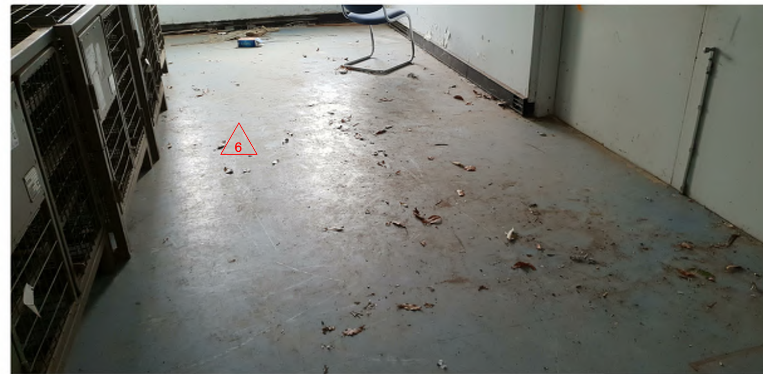
DAMAGED VINYL FLOOR SHEETING
