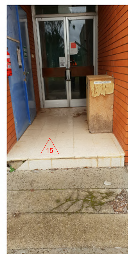
SCOPE 15 - TYPICAL CRACKED FLOOR TILES
