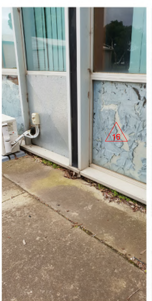
SCOPE 16 - CRACKED GLAZING TO BE REPLACED
