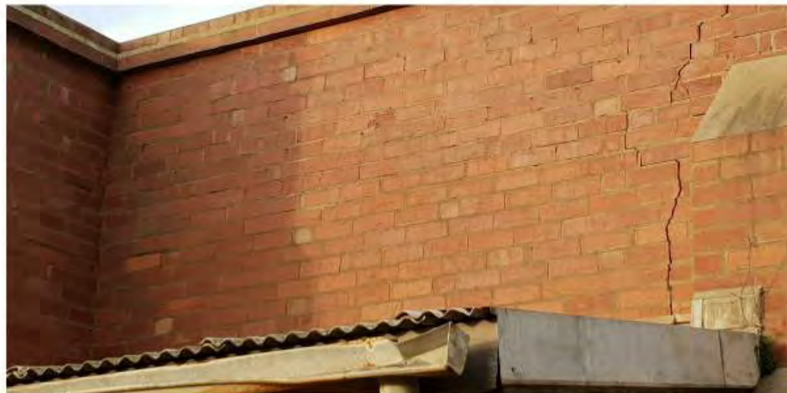
PHOTO NO 3 - VIEW OF SHED ROOF AND CRACKING IN WALL
