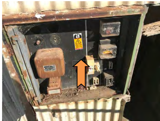
Photo 2. Asbestos-containing bituminous electrical board.
