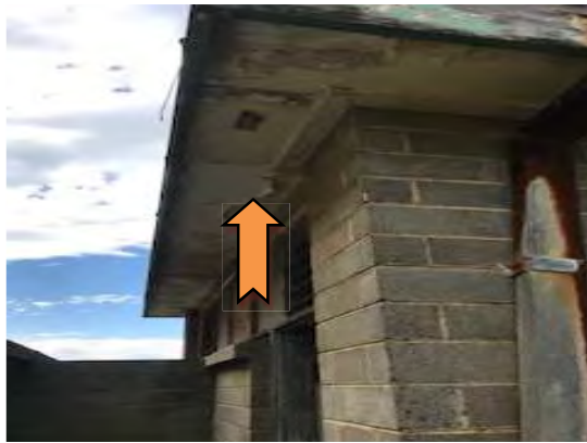
Photo 4. Asbestos-containing fibre cement sheet eaves.
