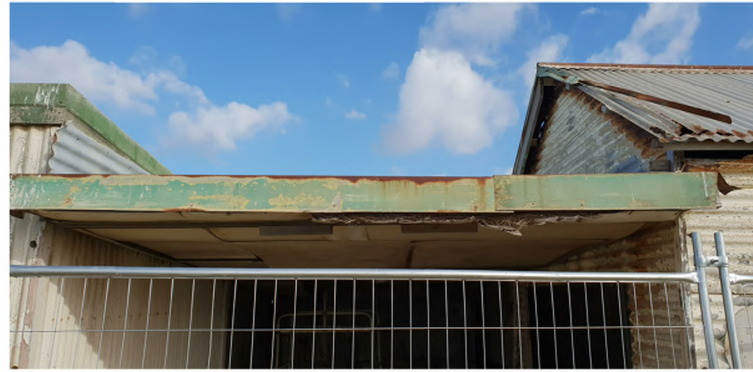
VIEW OF SOUTH ELEVATION - UNDERCOVER AREA - SHOWING FLASHING DETERIORATION
