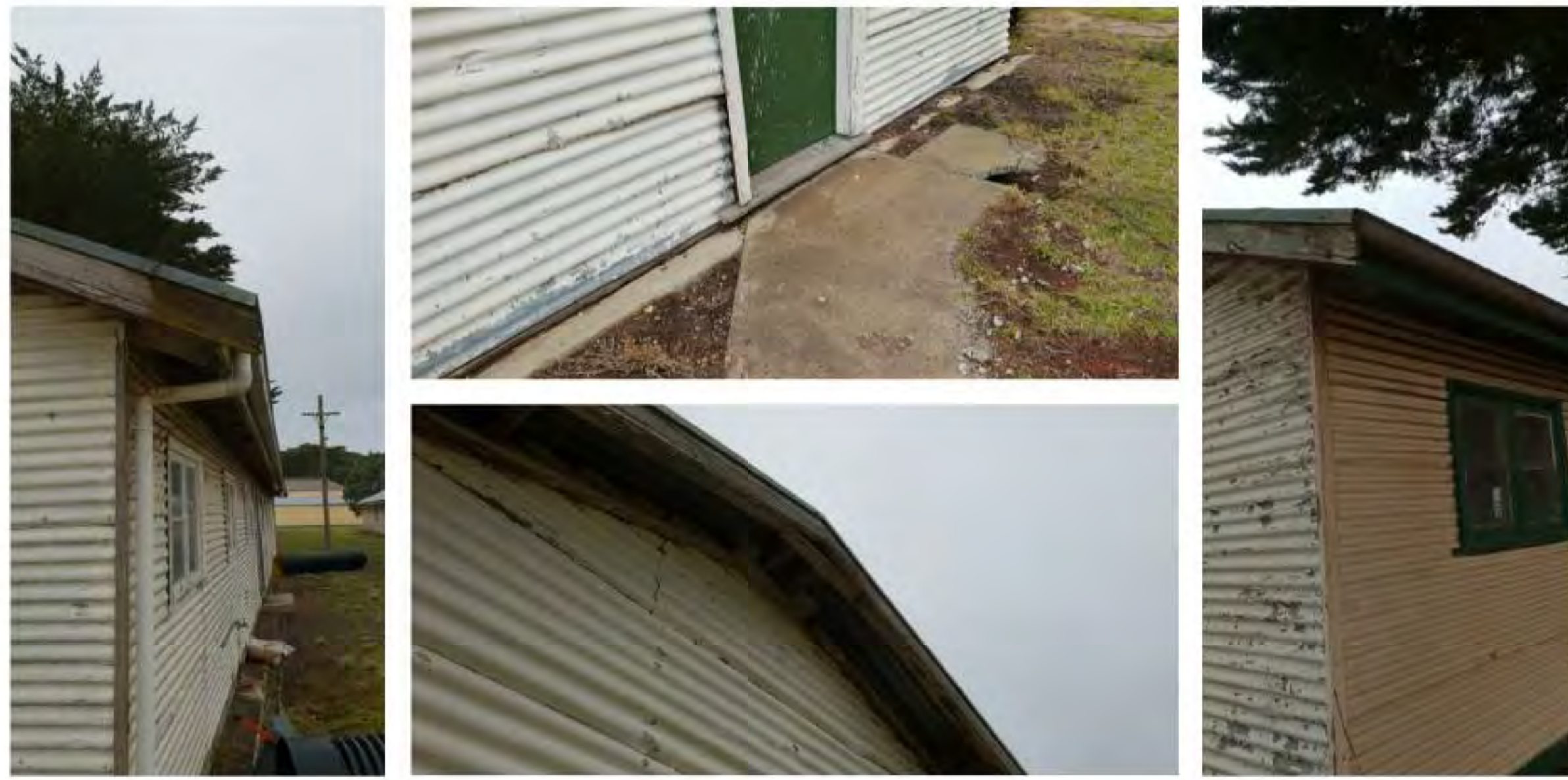
IMAGES OF TYPICAL DETERIORATION
