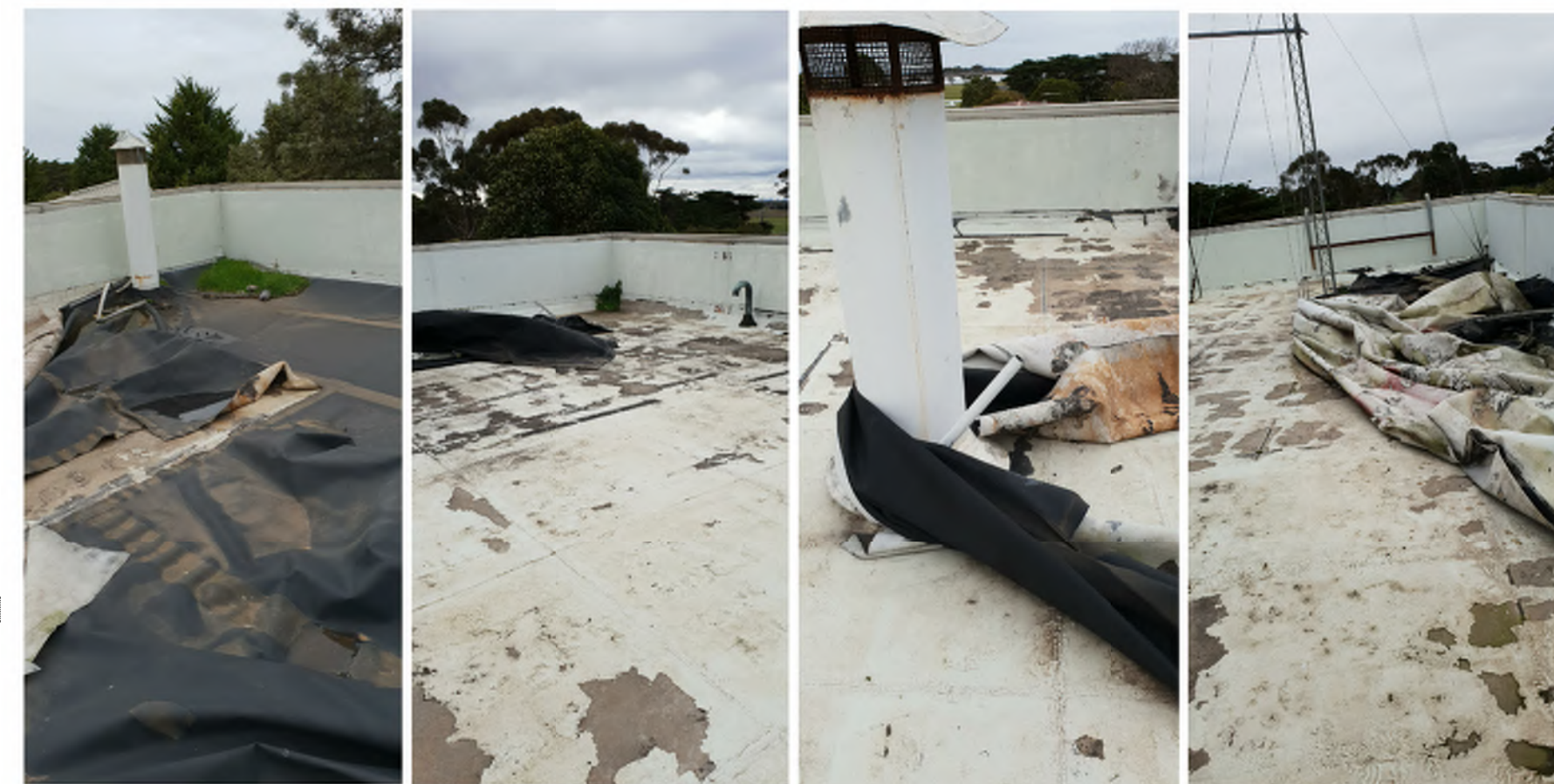
IMAGES OF DAMAGE TO WATERPROOF ROOF MEMBRANE
