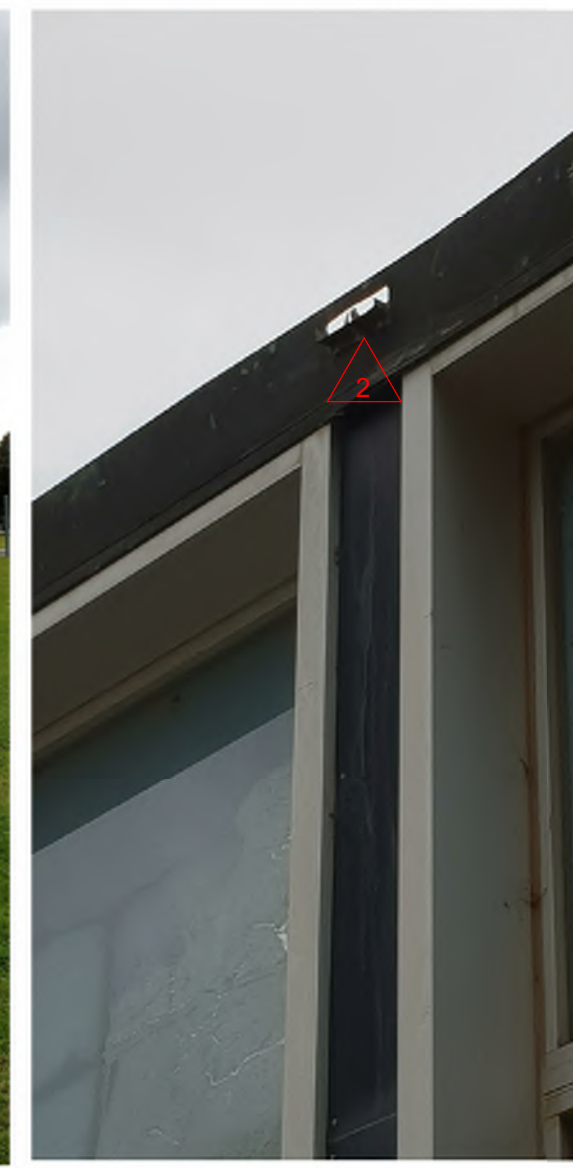
SCOPE 2 - IMAGE OF DAMAGED FLASHING
