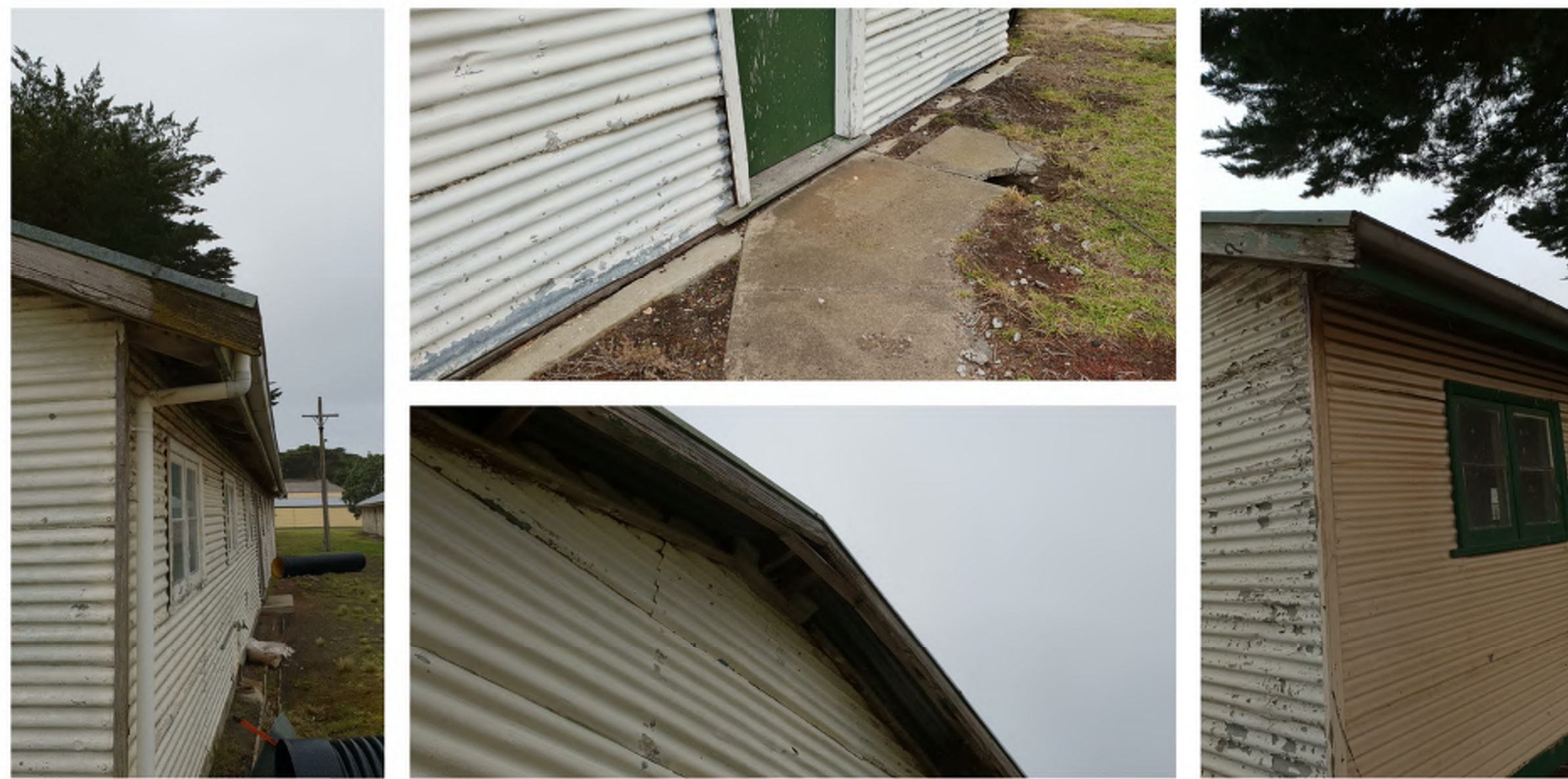
IMAGES OF TYPICAL DETERIORATION
