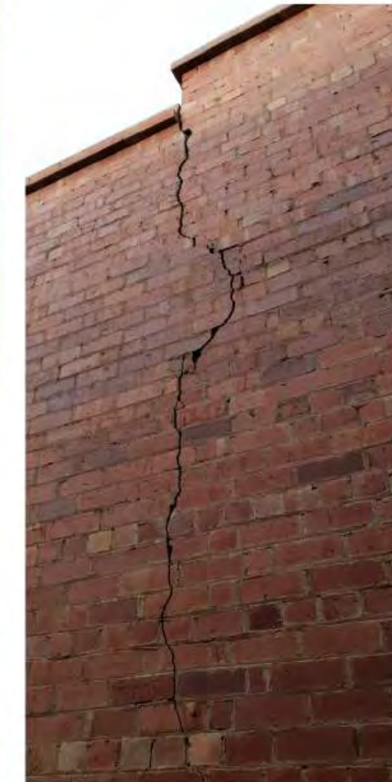
PHOTO NO 5 - VIEW OF CRACK IN WALL TO BE REPAIRED
