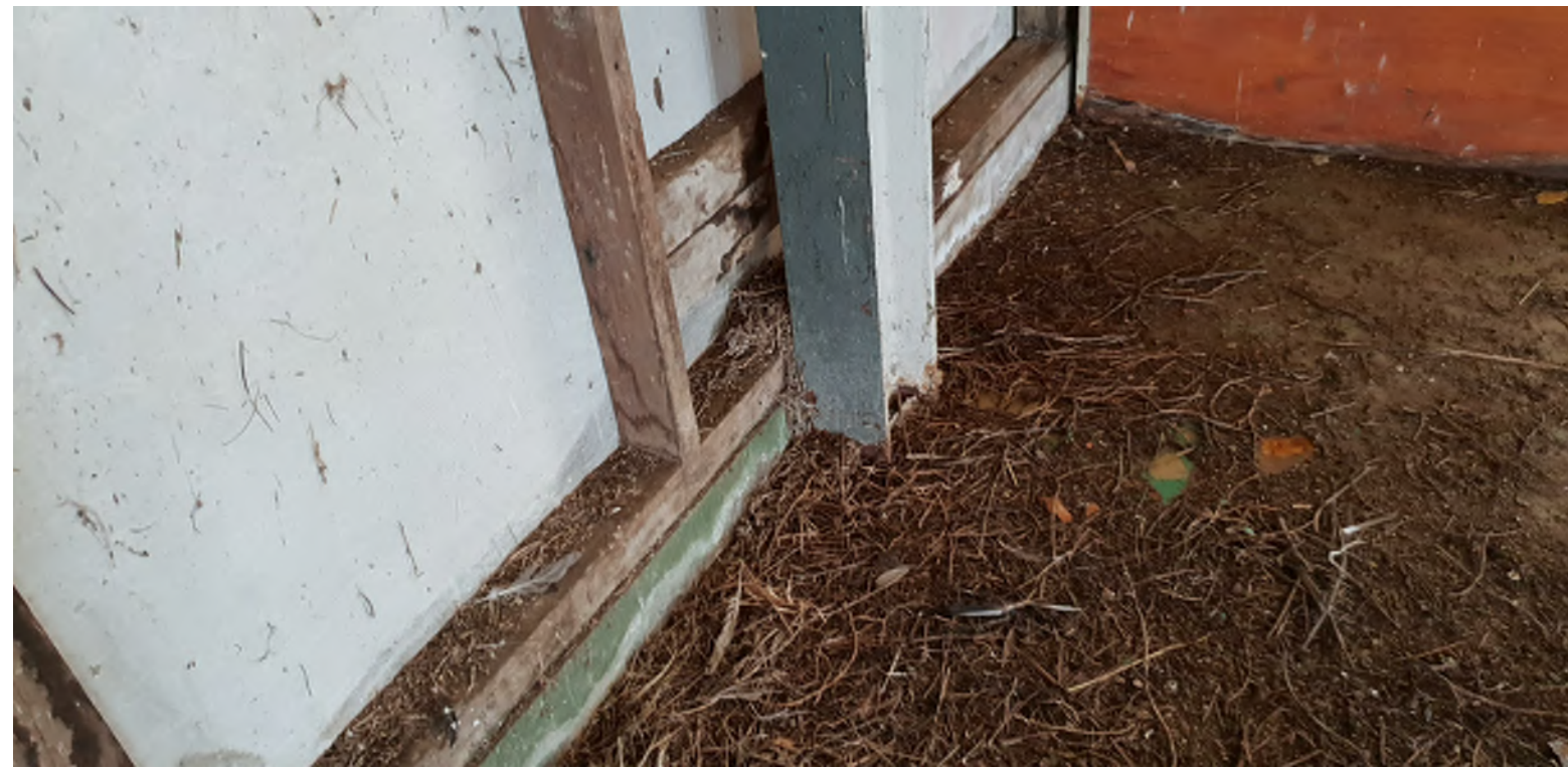
TYPICAL RUBBISH, LEAVES TO BE REMOVED FROM BUILDING
