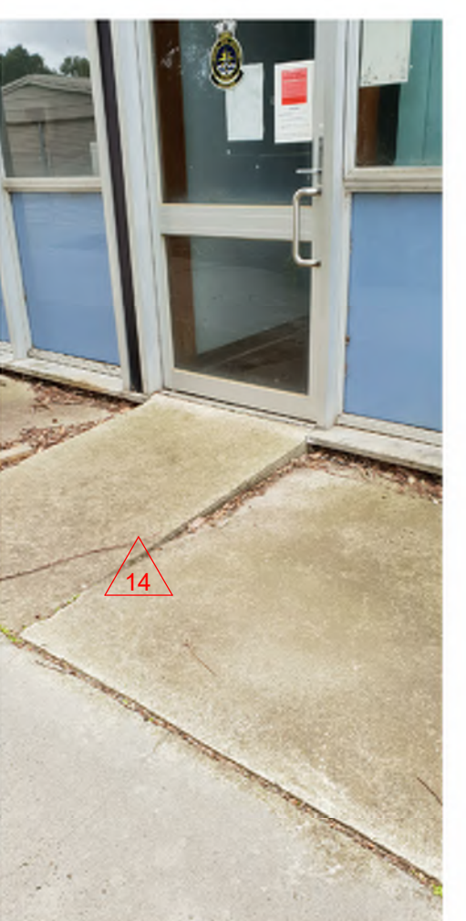
SCOPE 15 - TYPICAL CRACKED FLOOR TILES & PRESSURE CLEANED
