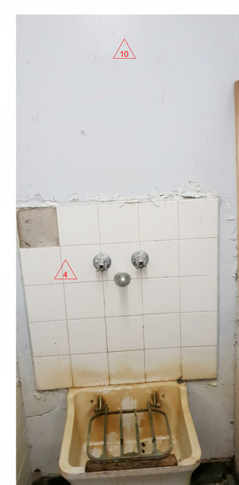
CLEANERS TROUGH DAMAGE
