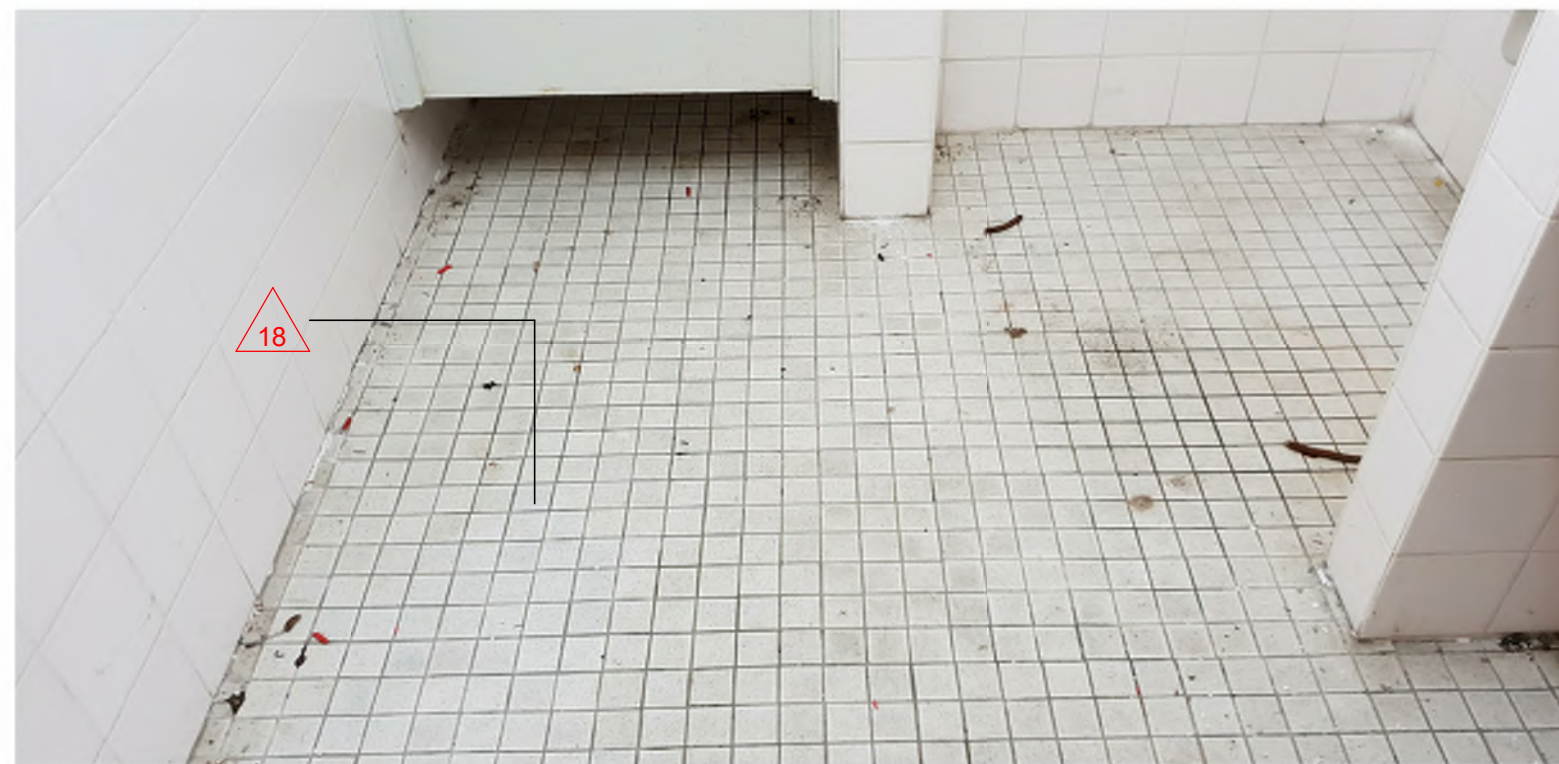
DAMAGED CERAMIC FLOOR AND WALL TILES
