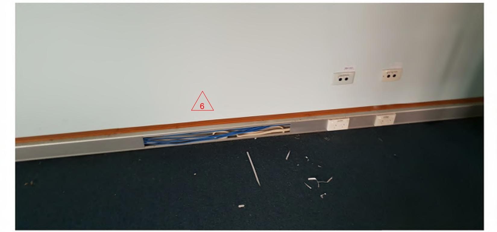
TYPICAL IMAGE OF DAMAGED INTERNAL SKIRTING FOR ELECTRICAL CONDUITS
