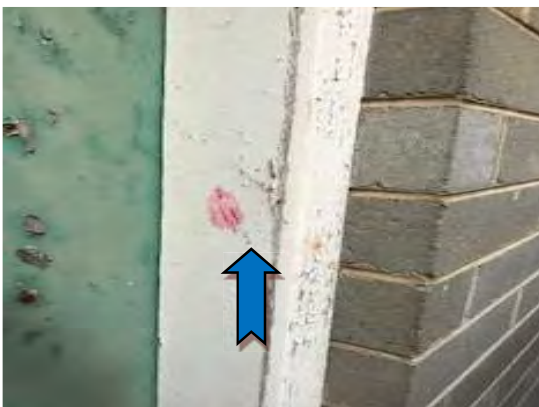
Photo 5. Lead-containing paints throughout the Site.
