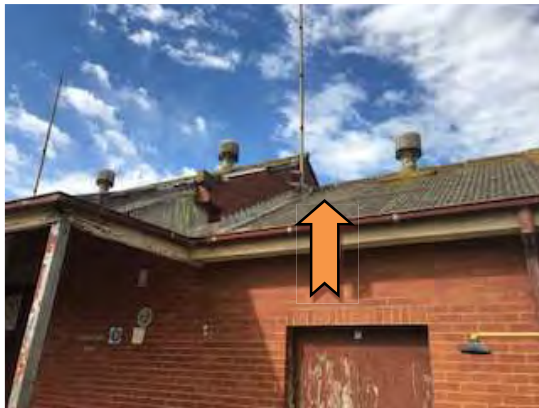
Photo 3. Asbestos-containing corrugated cement roof sheeting.
