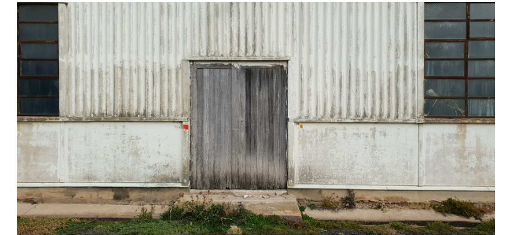
TYPICAL DETERIORATION OF EXTERNAL CLADDING AND TIMBER DOOR TO BE REPLACED
