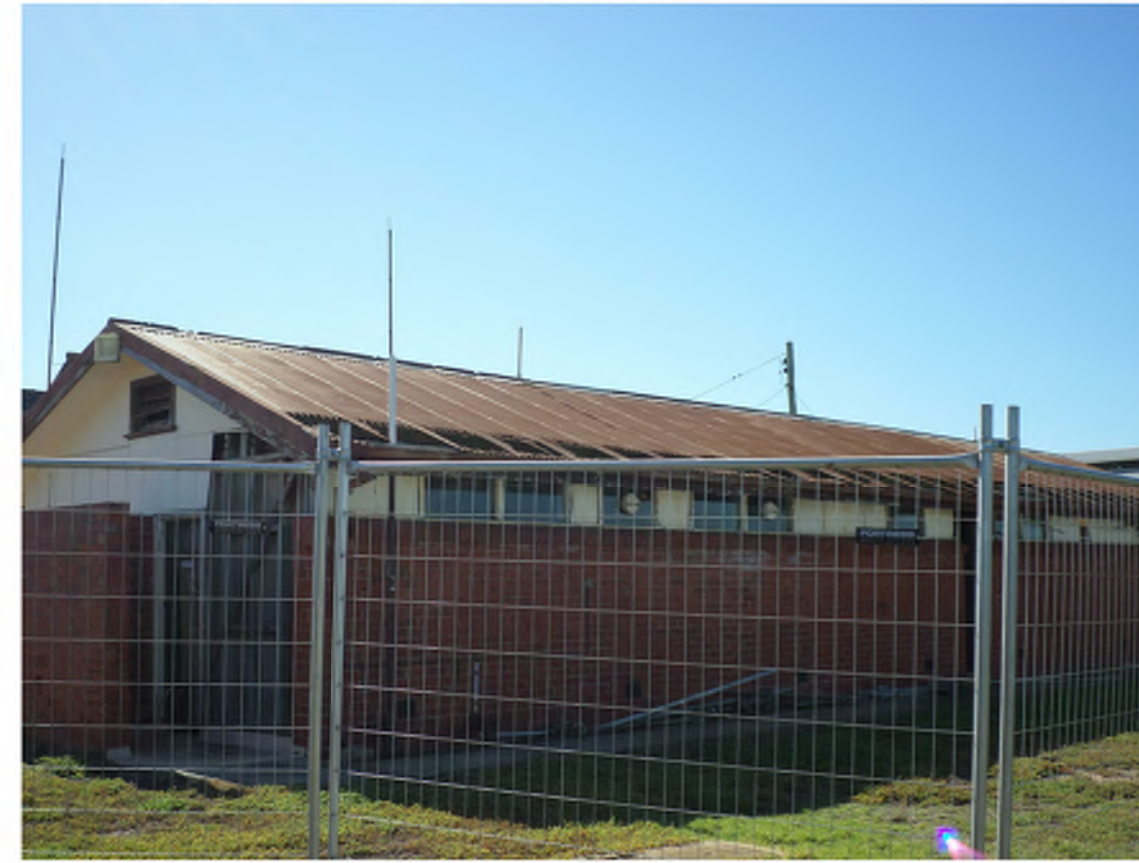
TOILET BLOCK SHOWING SIGNS OF DETERIORATION
