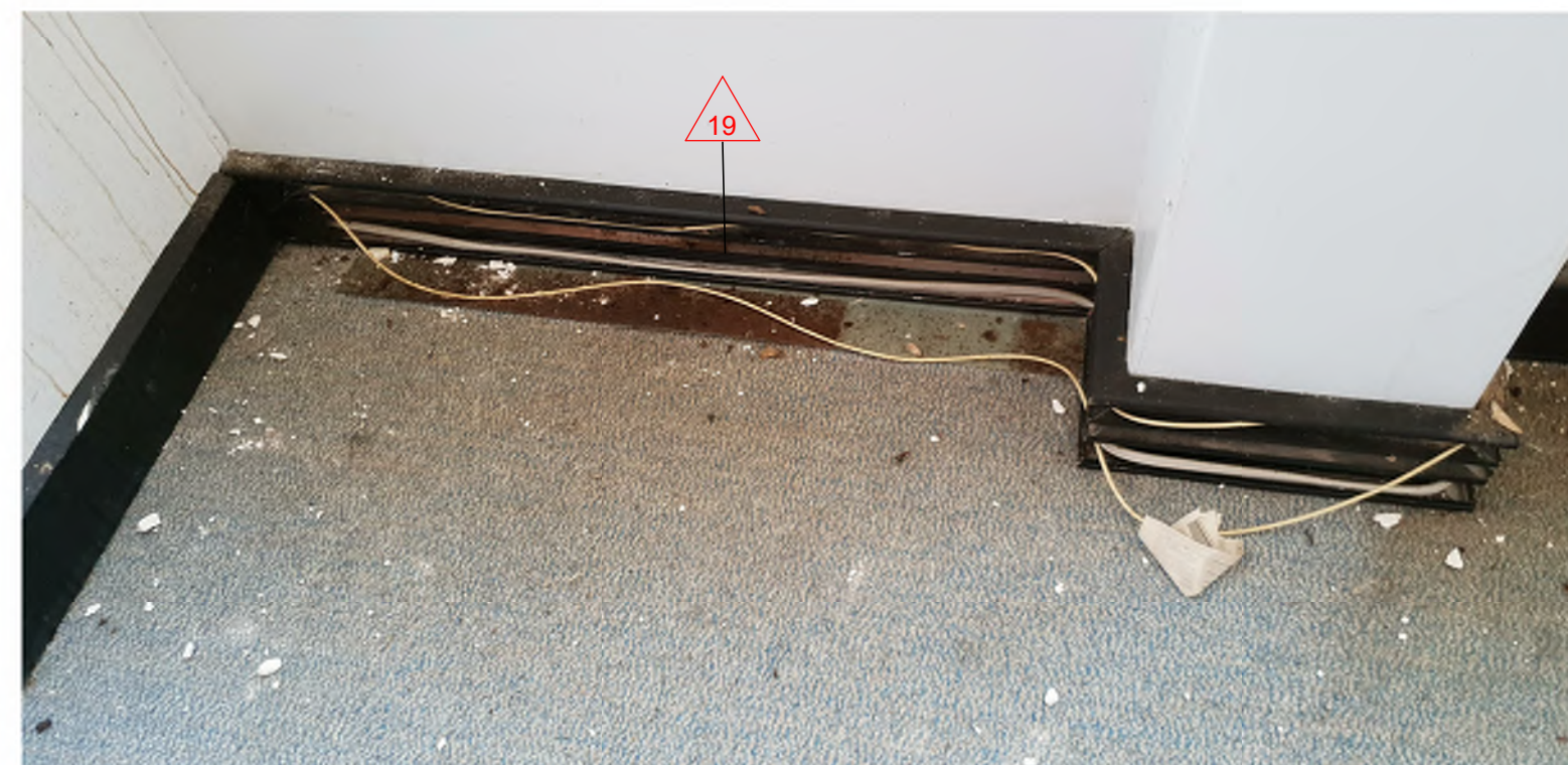
DAMAGE TO CARPETS AND SKIRTING DUCT
