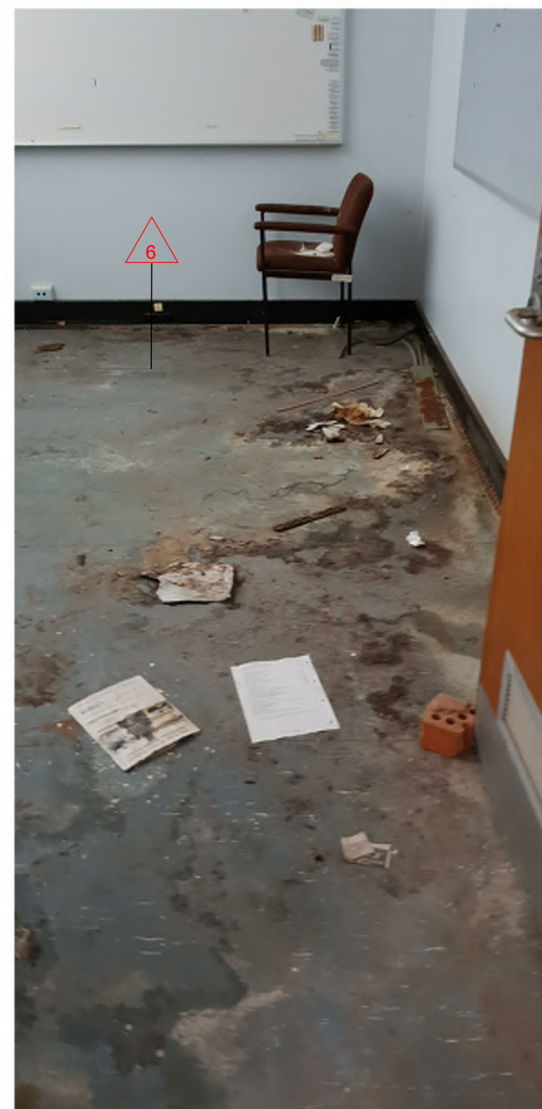
VINYL FLOOR SHEETING TO BE REPLACED
