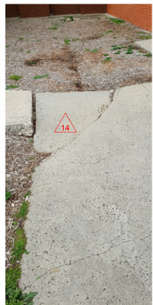
SCOPE 14 - TYPICAL CRACKED TILES
