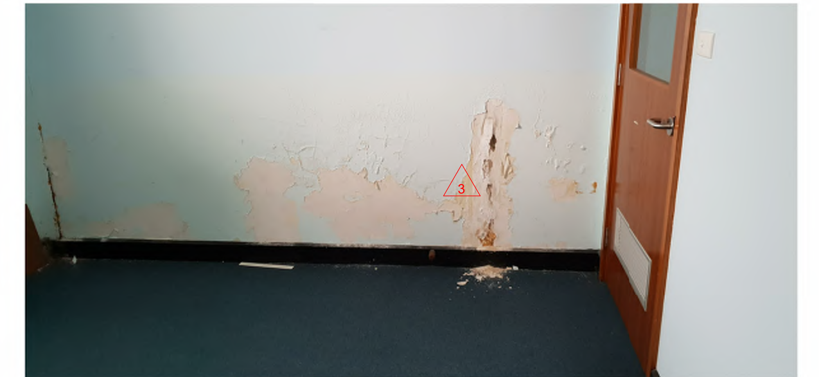
TYPICAL IMAGE OF DAMAGED WALLS
