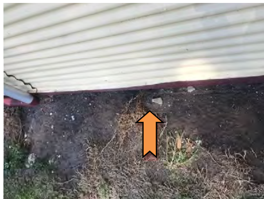
Photo 6. Asbestos containing fibre cement sheet debris to the external surface areas.
