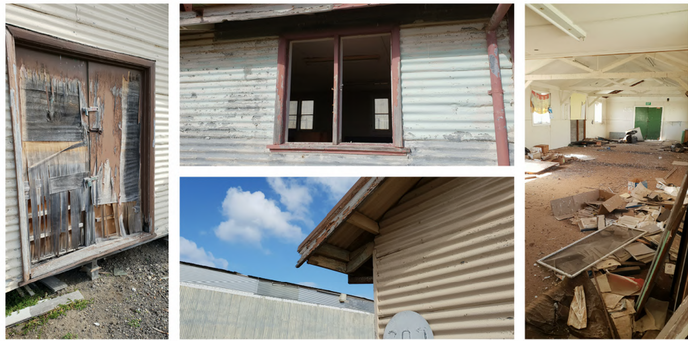
IMAGES OF TYPICAL DETERIORATION
