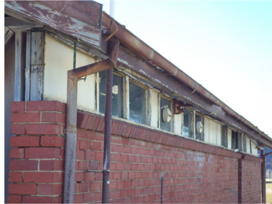
TOILET BLOCK SHOWING SIGNS OF DETERIORATION
