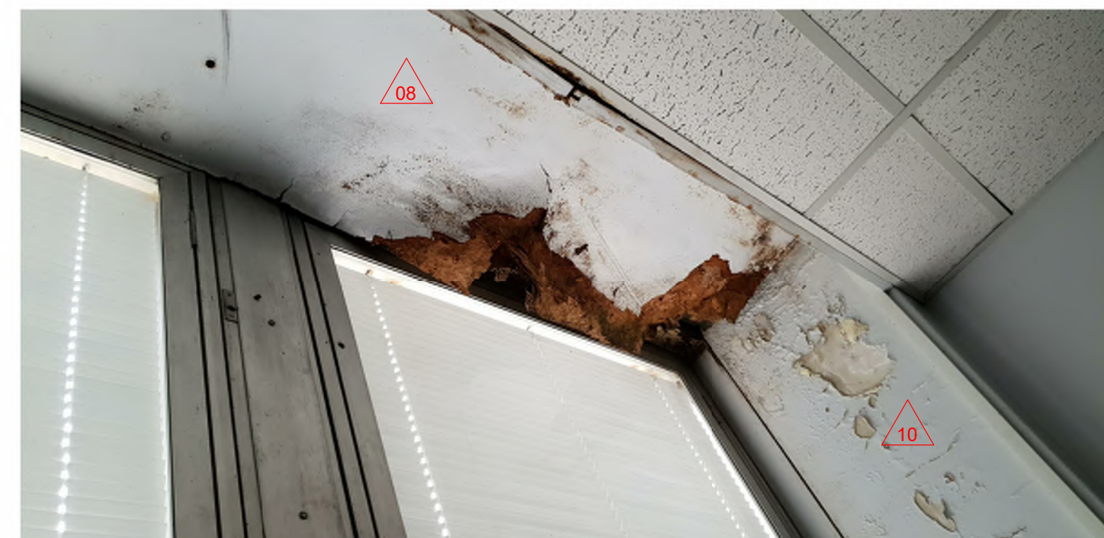
WATER DAMAGE OVER WINDOWS
