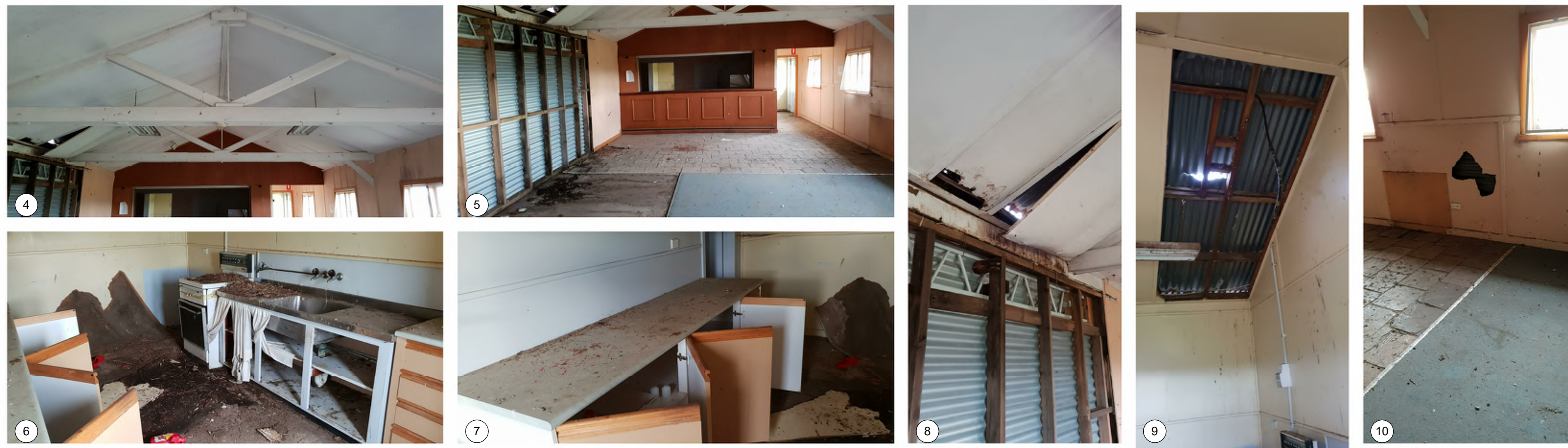
IMAGES OF TYPICAL DETERIORATION
