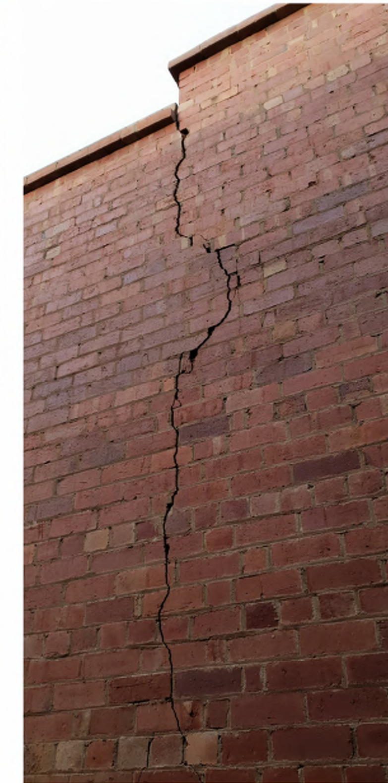
VIEW OF CRACK IN WALL
