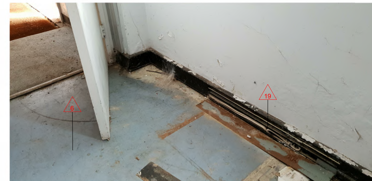
DAMAGE TO SKIRTING DUCT AND VINYL SHEETING
