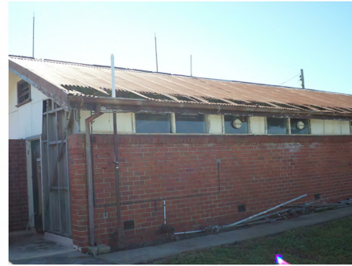
TOILET BLOCK SHOWING SIGNS OF DETERIORATION
