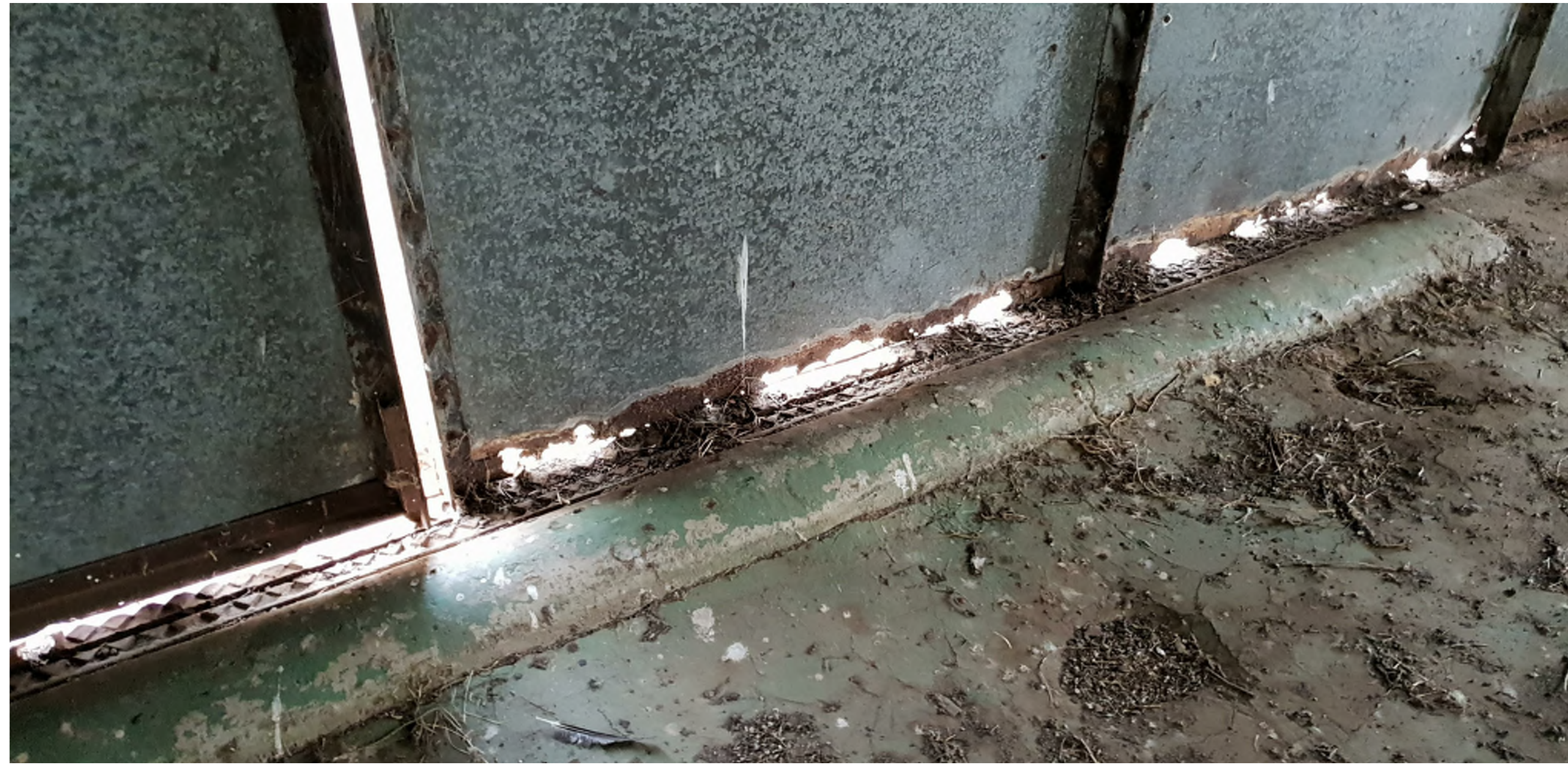
TYPICAL IMAGES - DAMAGE TO WALL LININGS
