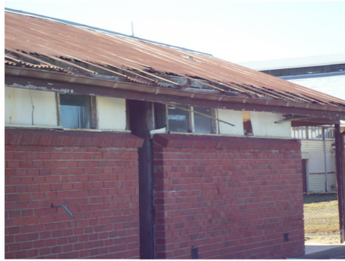
TOILET BLOCK SHOWING SIGNS OF DETERIORATION.
