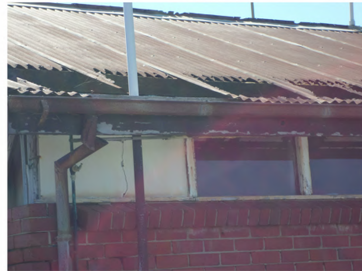
TOILET BLOCK SHOWING SIGNS OF DETERIORATION
