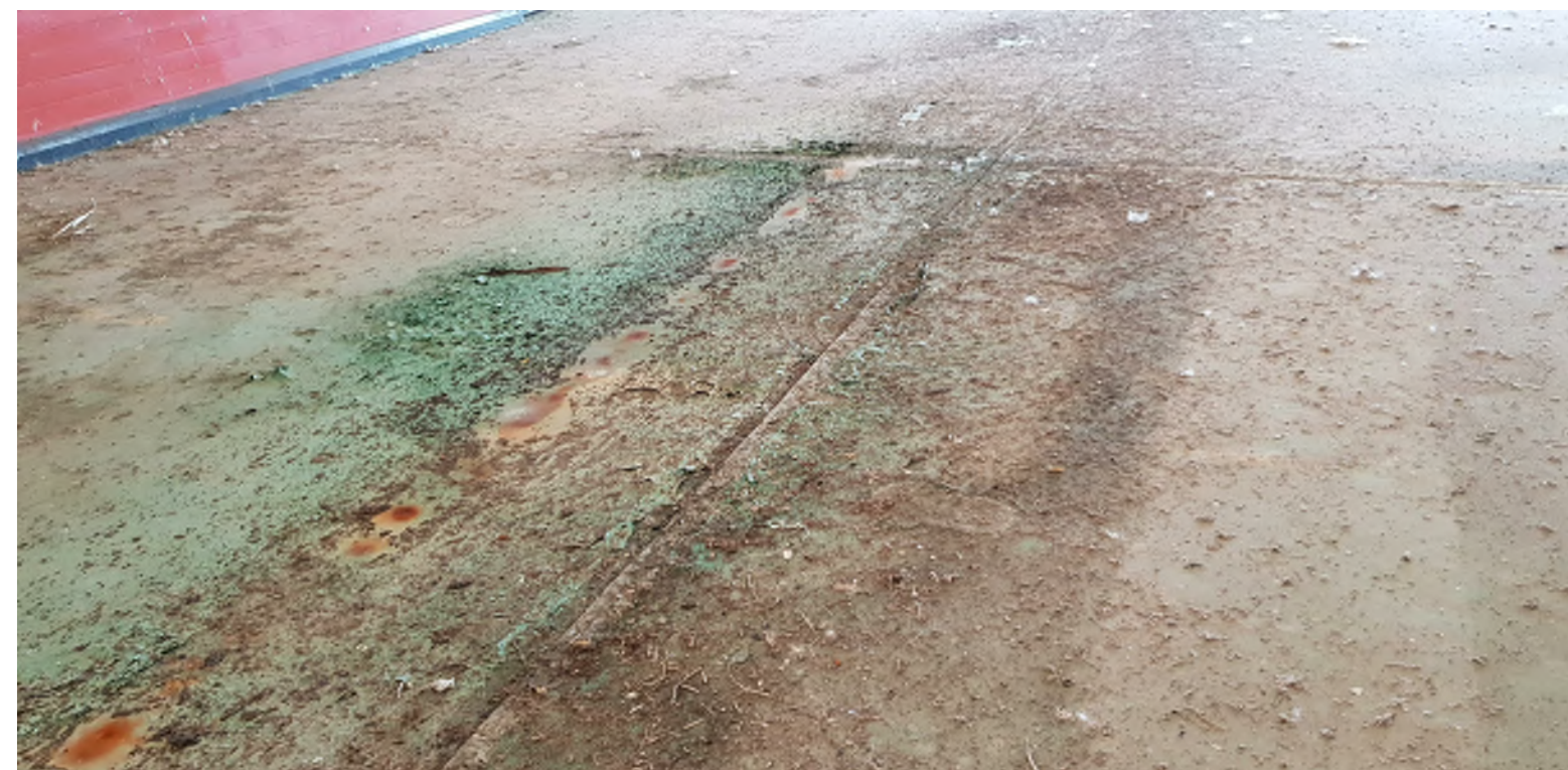
TYPICAL CONCRETE SLAB - SHOWING EXTENT OF DIRT BUILD UP TO BE REMOVED
