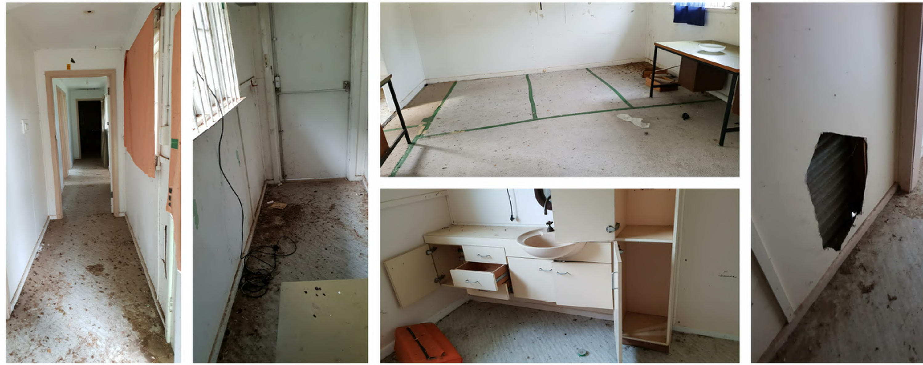
IMAGES OF TYPICAL DETERIORATION
