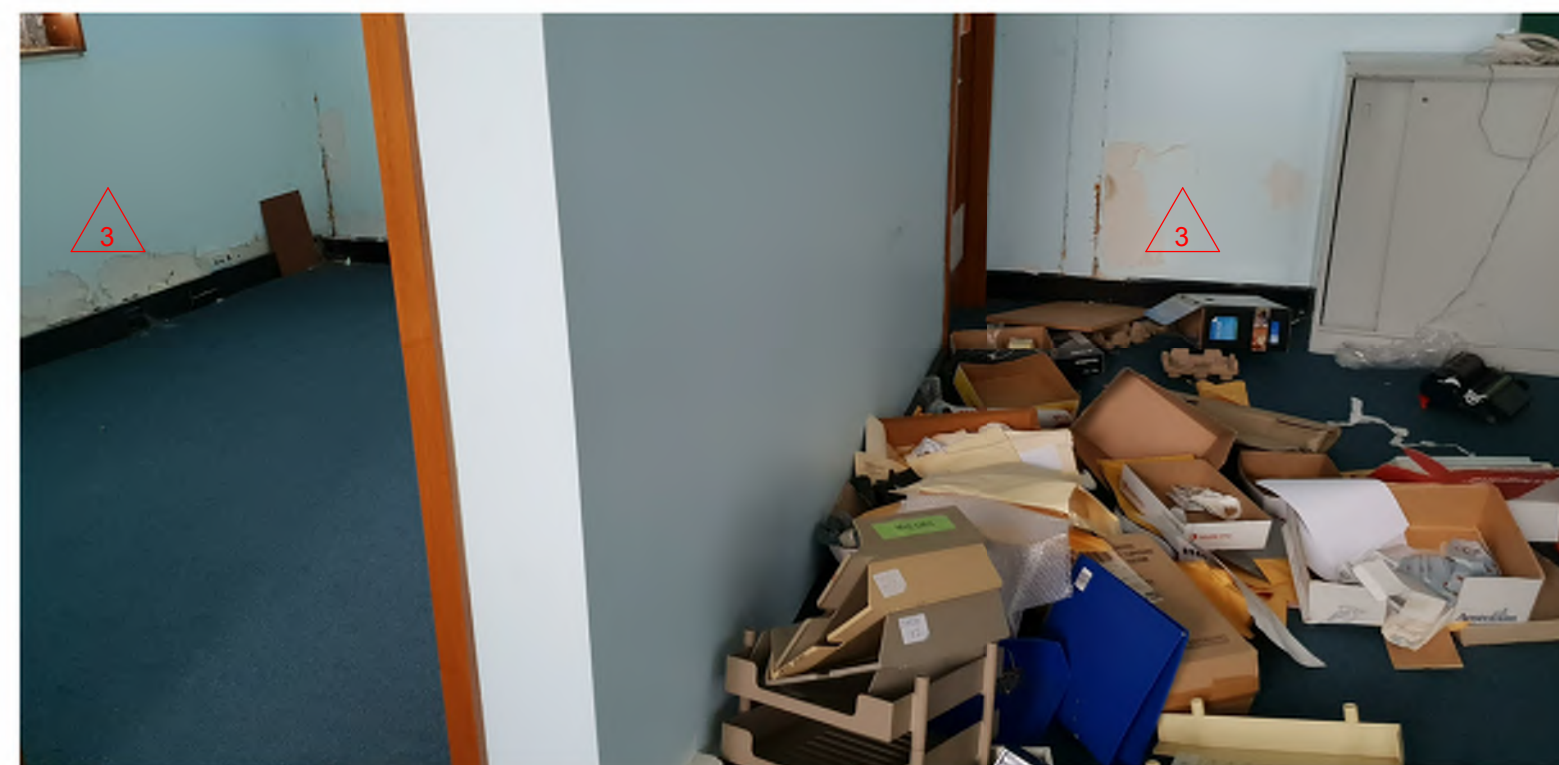
TYPICAL INTERNAL WALL DAMAGE AND LOOSE FURNITURE DEBRIS WITHIN THE OFFICES
