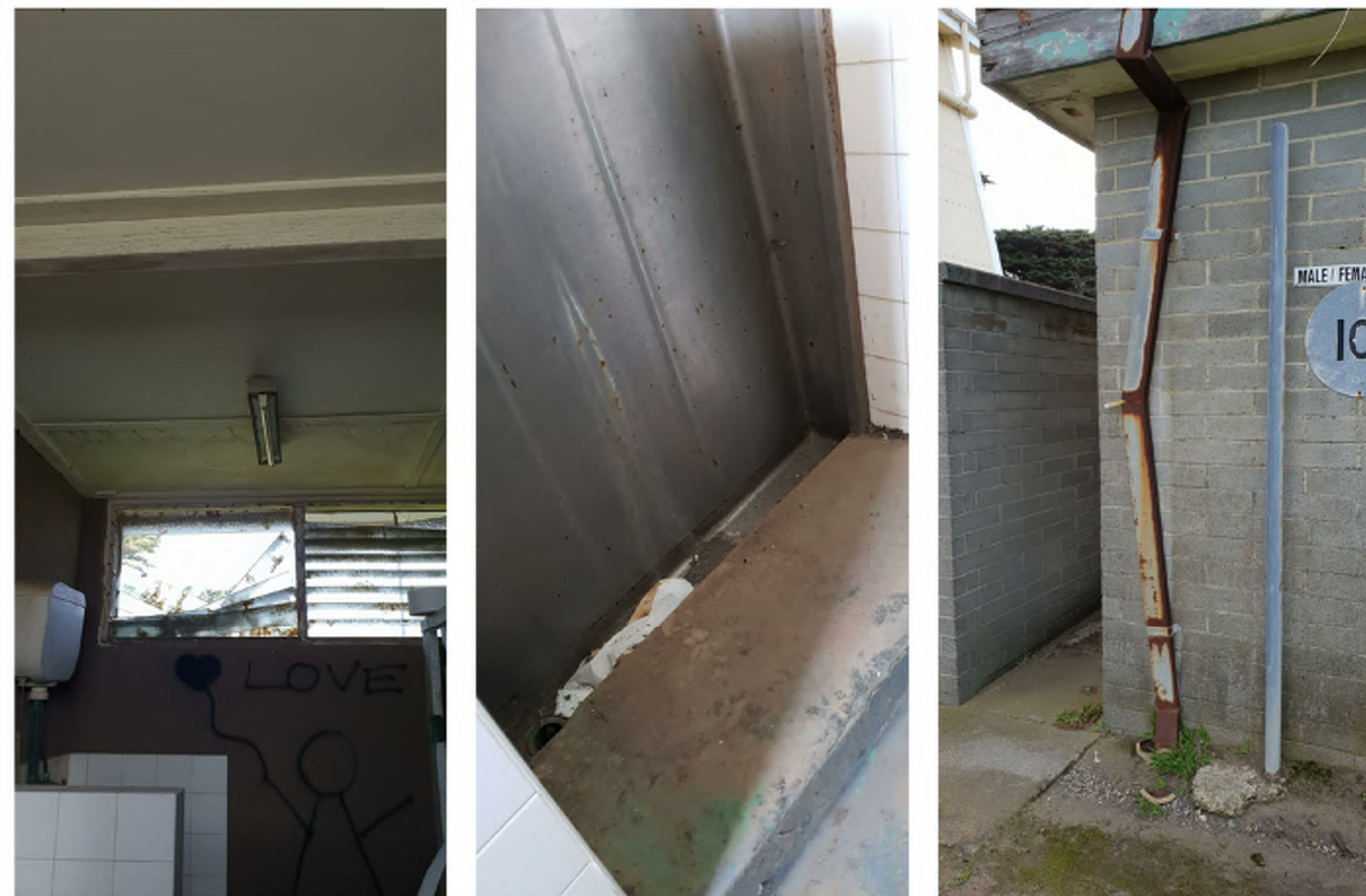
IMAGES OF TYPICAL DETERIORATION
