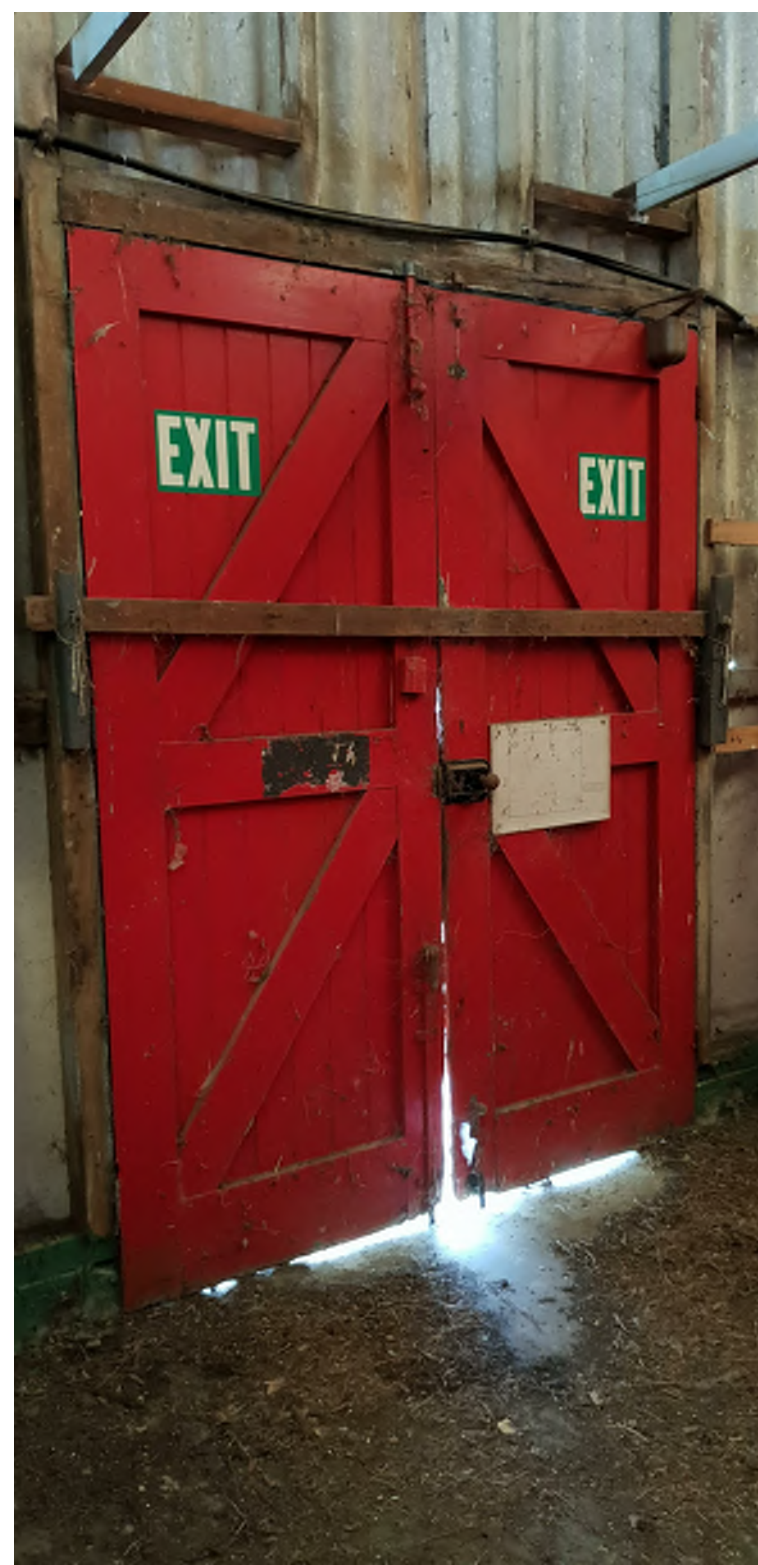
EXISTING DOORS TO BE REPLACED
