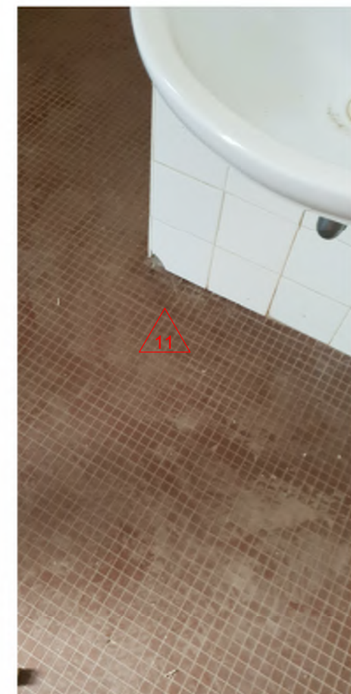
SCOPE 8 - IMAGE OF BATHROOM TILES NEED REPLACEMENT
