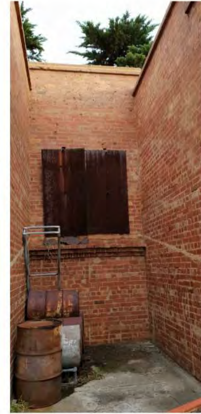
PHOTO NO 4 - VIEW INTO THE STRUCTURE, SHOWING RUSTING SHEET PANELS
