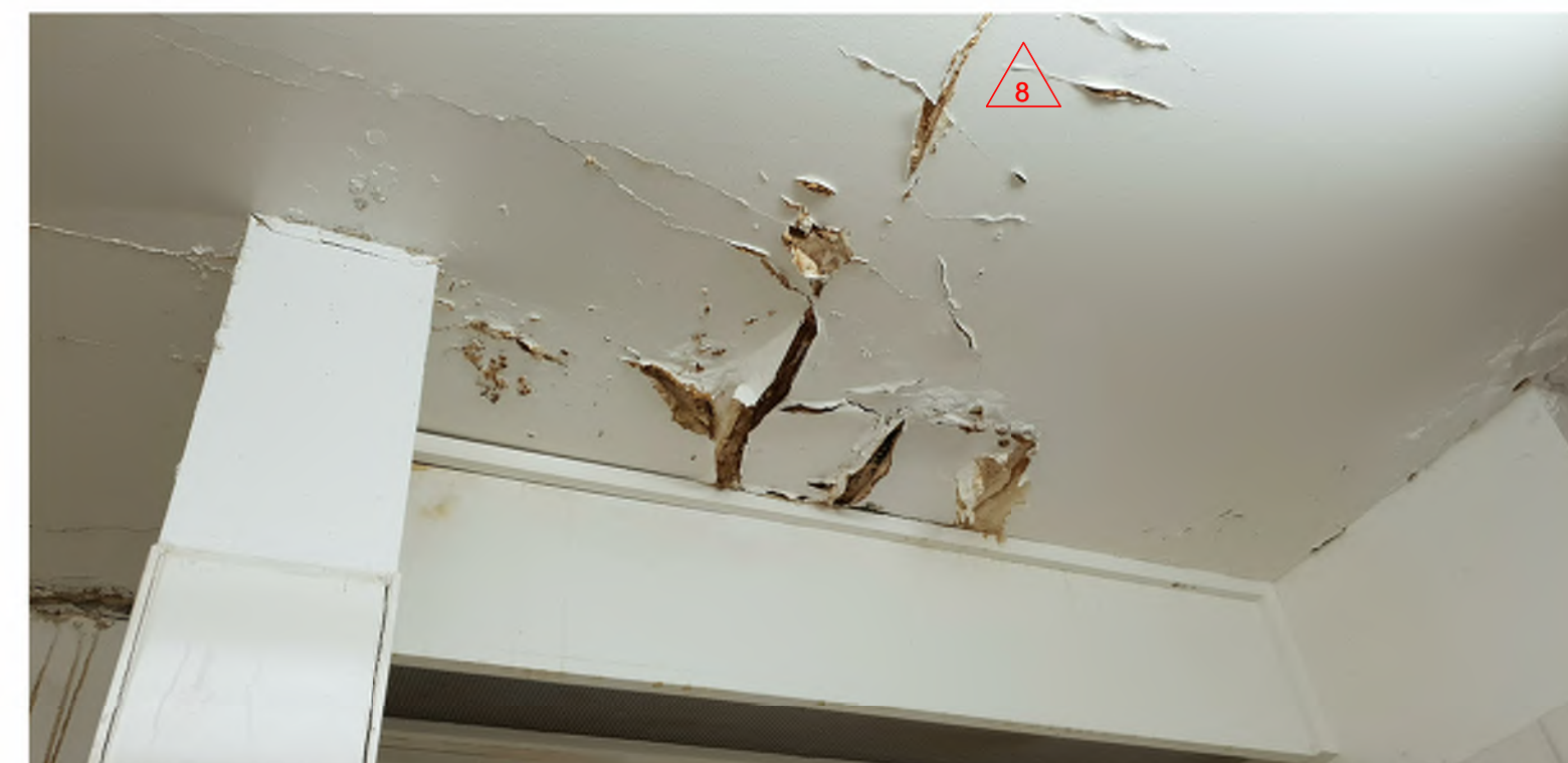
TYPICAL WATER DAMAGE TO CEILINGS
