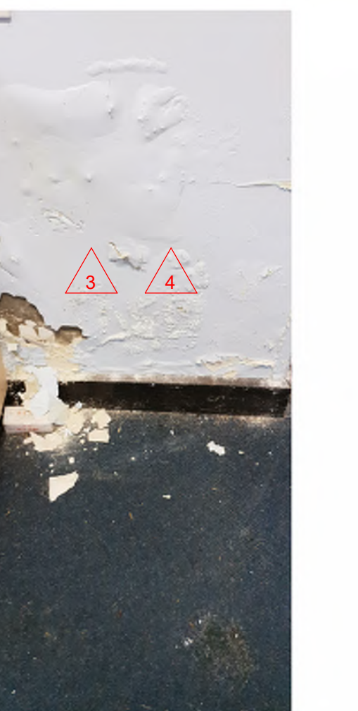
TYPICAL INTERNAL WALL DAMAGE
