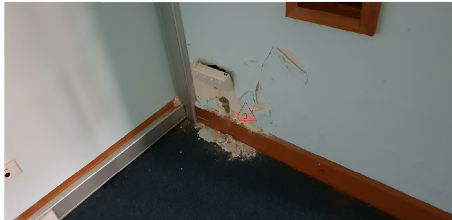
SCOPE 3 - IMAGE OF TYPICAL INTERNAL WALLS DAMAGE TO BE PATCHED AND PAINTED
