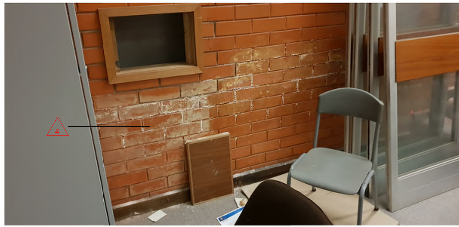
SCOPE 4 - IMAGE OF TYPICAL WATER DAMAGE TO MASONRY WALLS
