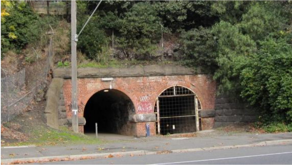
Figure 39 Pedestrian and creek tunnels, east end of railway reserve, as seen off Scott Parade
