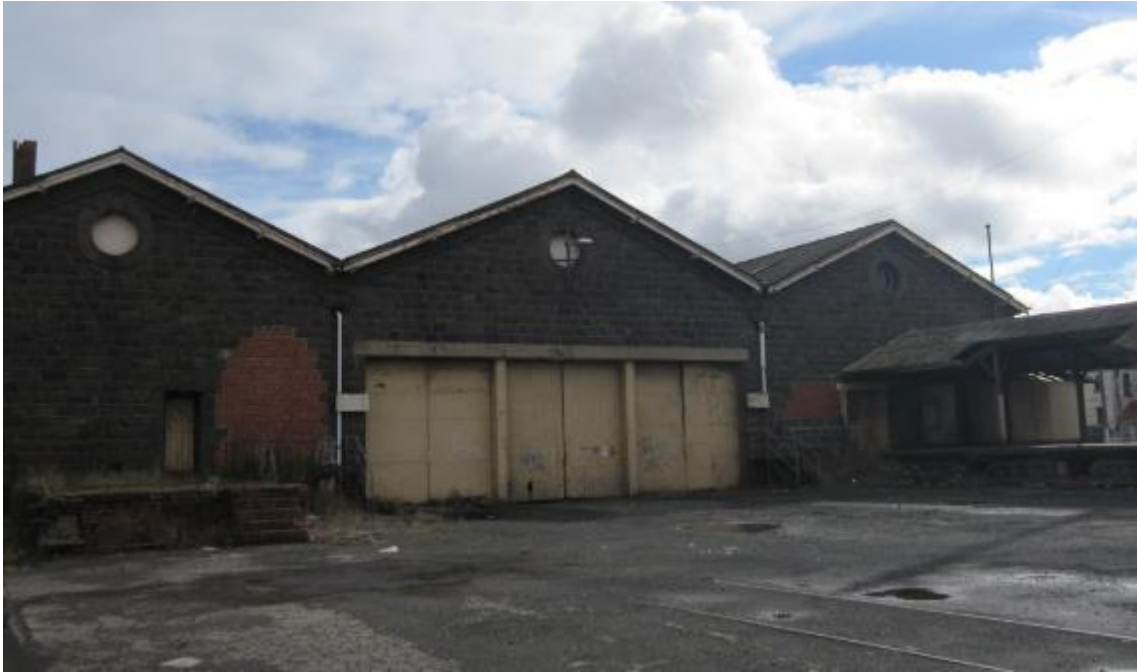
Figure 11 Another view of the east elevation; the underground facility is located beneath the short section of platform extending from the elevation, at left; this section of platform is proposed for removal.
