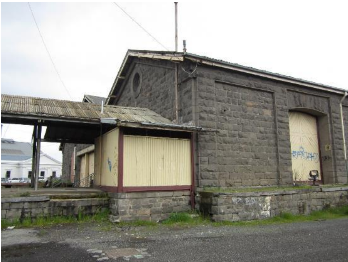
Figure 10 East end of Goods Shed; the platform off the gabled end, enclosed structure and posted awning are proposed for removal
