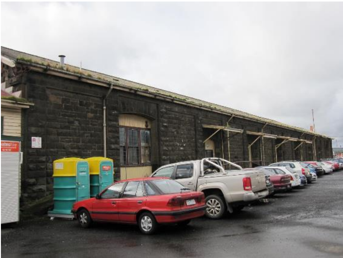
Figure 6 South elevation; the awnings are proposed to be retained and refurbished; the large opening at centre is proposed to be infilled with new aluminium-framed glazing
