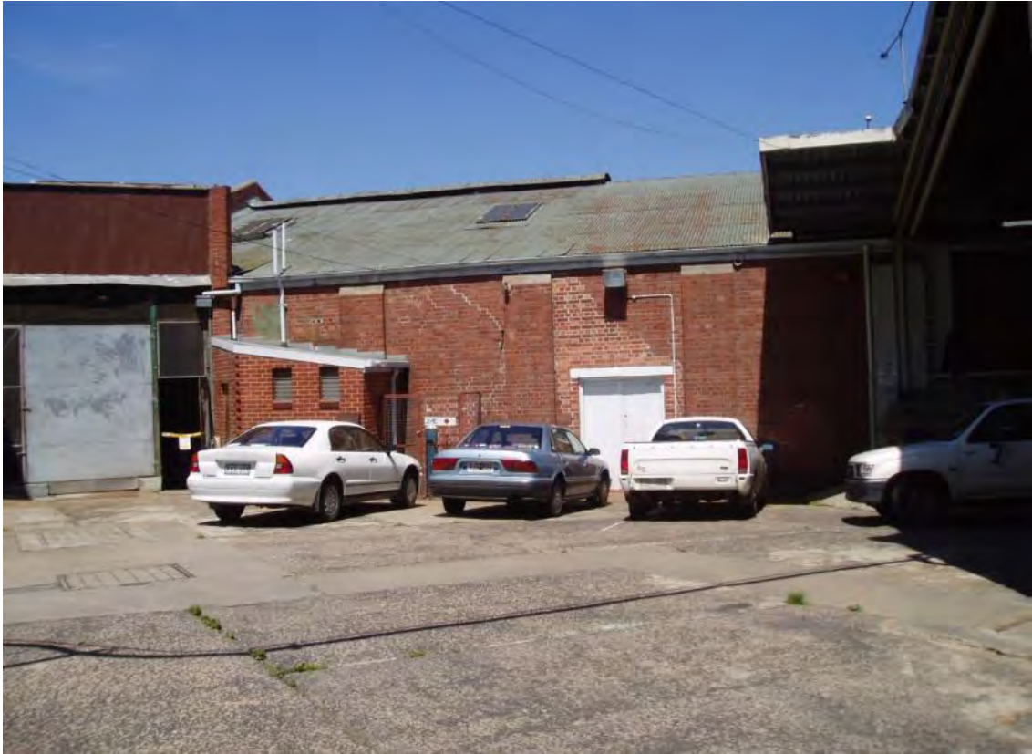
Figure 32 B6, east end, showing section of north wall and roof; this building component is being retained, excluding the addition at left and the adjoining minor brick annex
