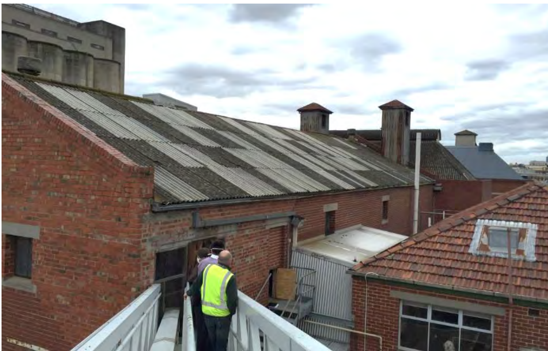
Figure 18 B4 roof with the kiln towers visible, and the south end gable at left; B3 is at right
