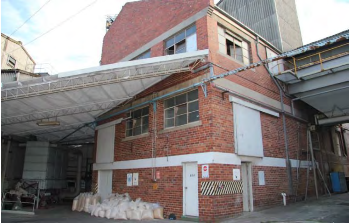
Figure 22 B5, south end, showing 1930s extension; the steel awning at left will be removed; the ground floor level walls will also be substantially removed
