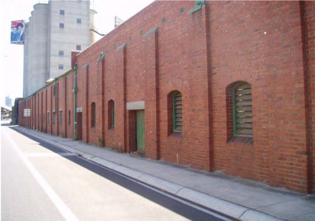
Figure 30 B6, south elevation to Harcourt Parade, with the wall of the 1928 east addition at right; this elevation will be retained
