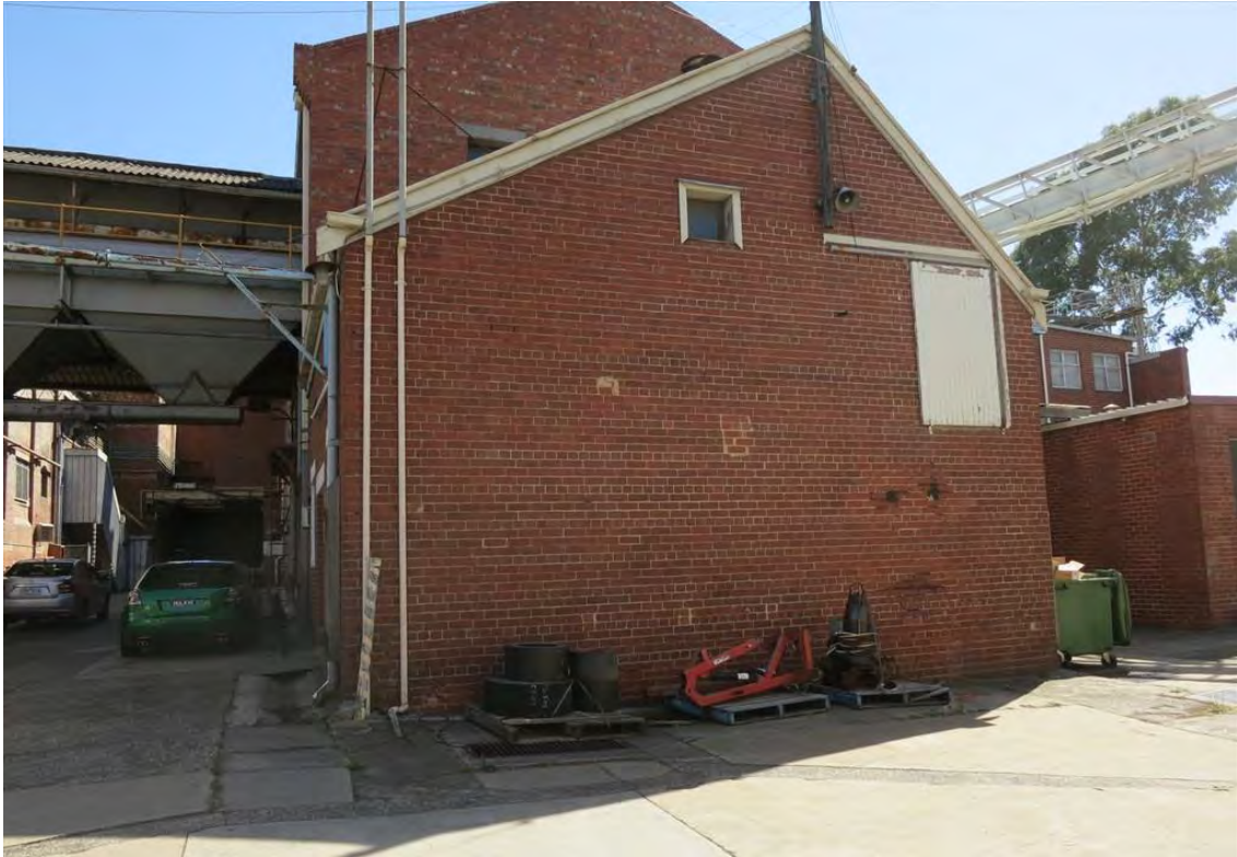
Figure 15 Rear of B4, showing the south end gabled bay proposed for removal
