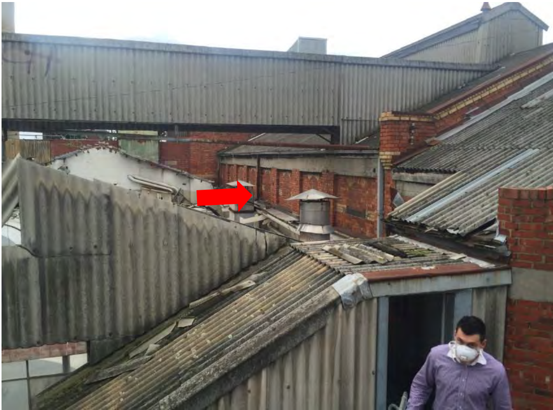
Figure 24 View to top level and roof of B5, showing part of the original 1880s bichromatic brick west elevation (indicated)
