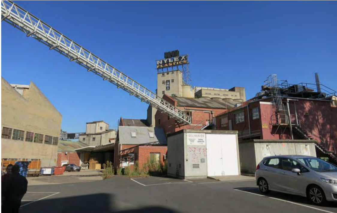
Figure 10 Internal view of east end of site, looking west: structures in the foreground are proposed for removal; B3 is at right, with the visible building component proposed for demolition
