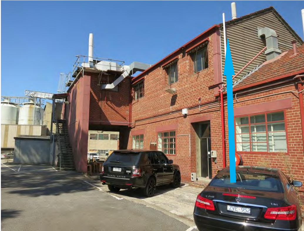
Figure 13 B3: the building component to left of the blue arrow, including the porte cochere and remnant of the west wall of the 1903 malt house, are proposed for removal
