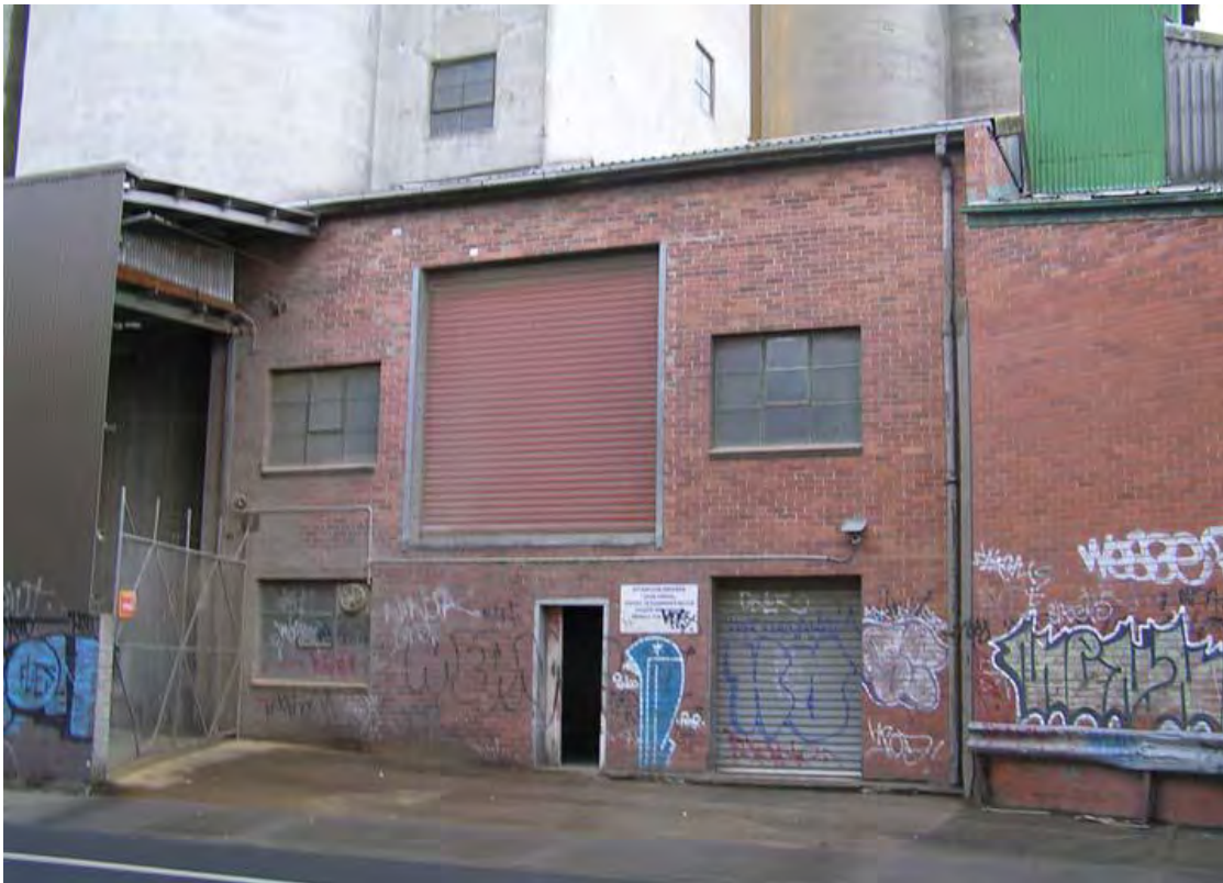
Figure 31 B6, western addition, showing the south elevation to Harcourt Parade; this component is proposed for demolition
