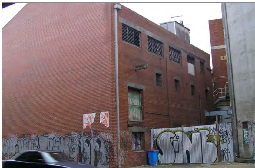
Figure 49 B11, non-original south elevation at left, and east elevation at right (as seen from Harcourt Parade)
